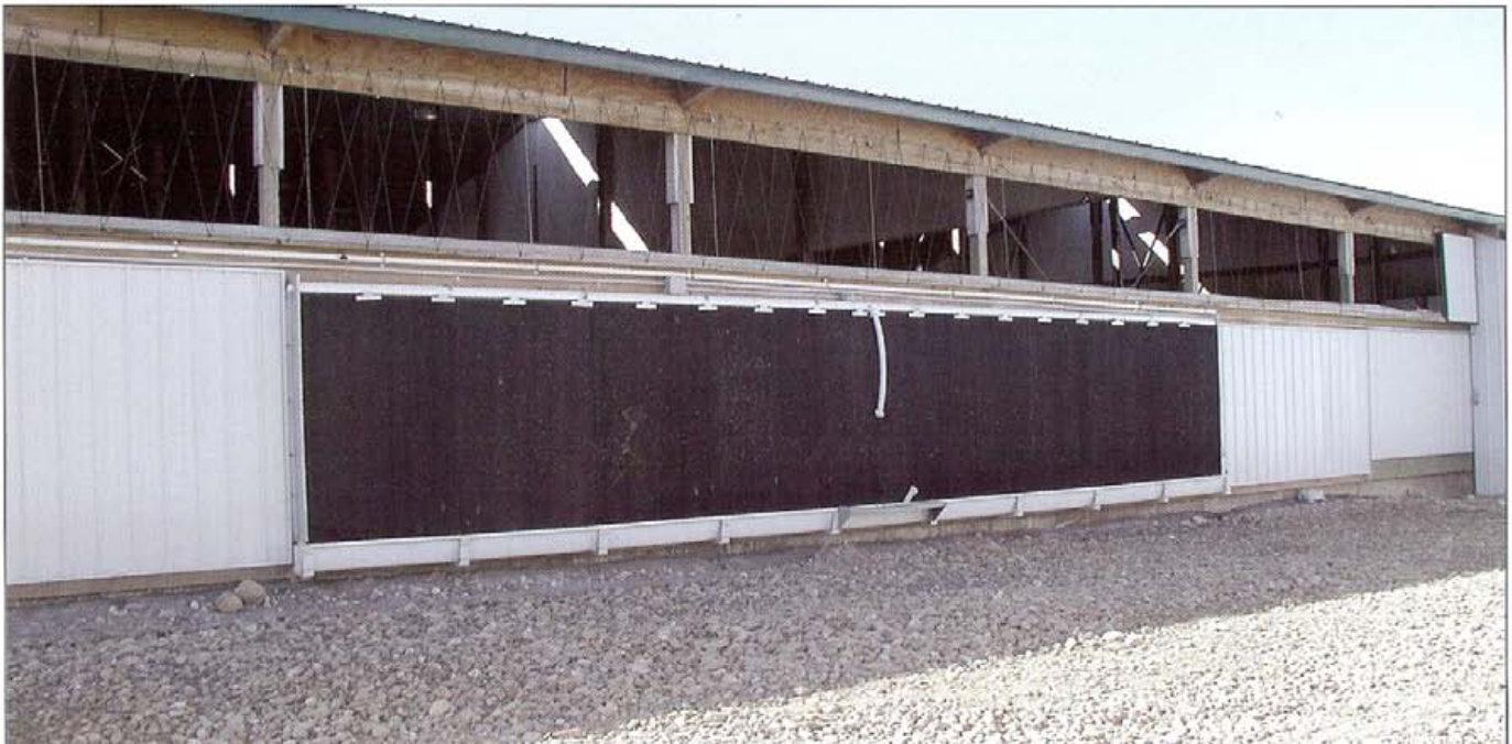
Pro-Kool Evaporative Cooling System
